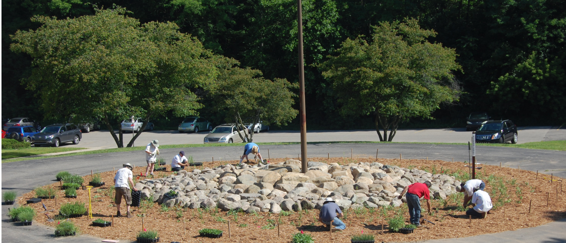
A landscaping crew and Wild Ones volunteers begin planting over 2000 native wildflowers and grasses in front of the Kalamazoo Public Schools administration building on Howard Street
